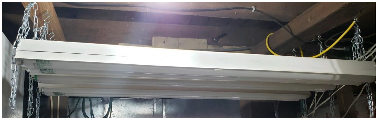
Lighting Fixture Photo by mrl2022
